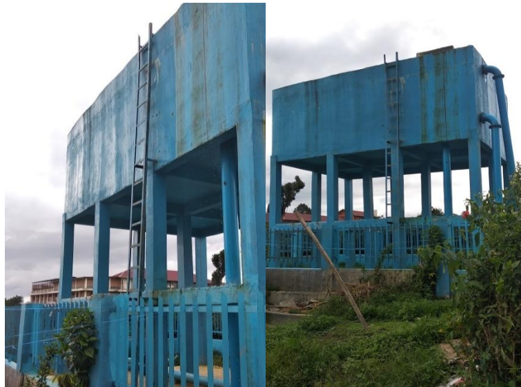
Gambar 2.3.4 Reservoir Jl. Garuda Aek Bolon Kap. 50 m 3
